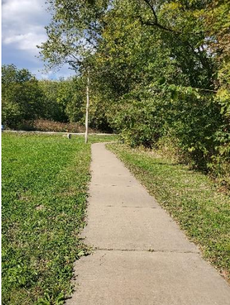
Good : Unlikely to hinder mobility of the average pedestrian. The sidewalk is free from significant cracking, buckling, gravel surfaces, or other debris which would impede pedestrian traffic.
